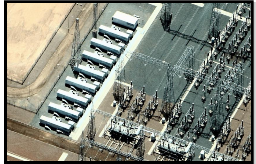
Site: 12 MW, Los Andes substation, Atacama Desert
