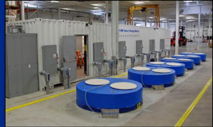
First MW inside
