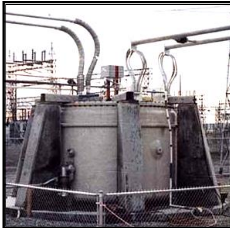
10 MW – 3 Sec. Coil Tested For Transmission Stability Bonneville Power Administration
