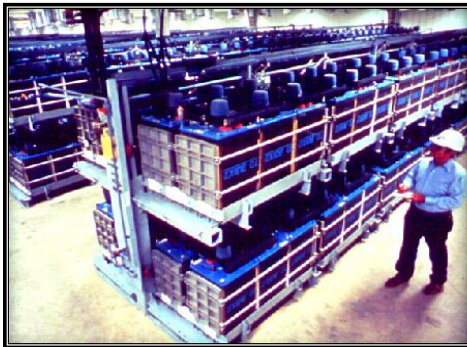
10 MW – 4 Hr Lead Acid Battery Plant At Southern California Edison (1988)
