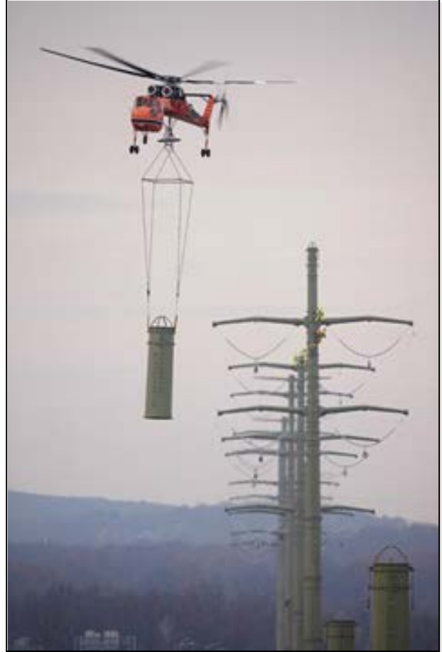
Susquehanna Roseland Project
